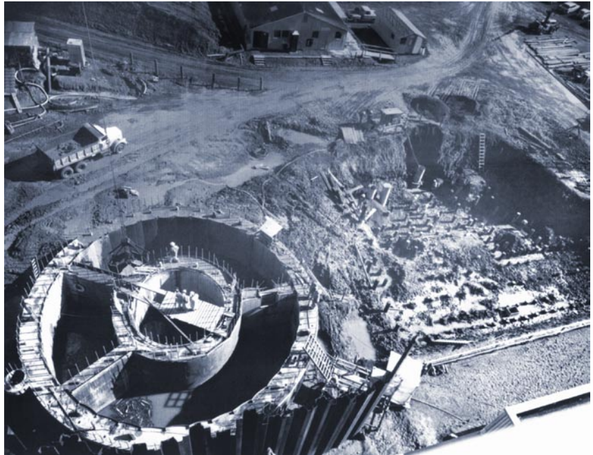
Aerial view showing construction of the concrete caisson for the nuclear reactor.
