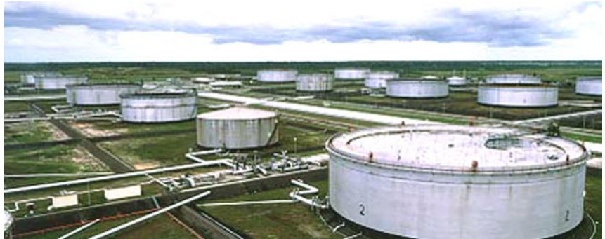
Tank farm at Bonny Island, Nigeria.
