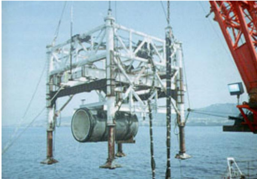
First replacement concrete pipe section during lowering with "horse" at Point Loma.
