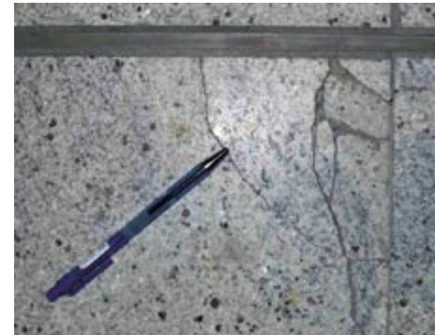
Cracked granite floor due to low strength granite and poor grouting.
