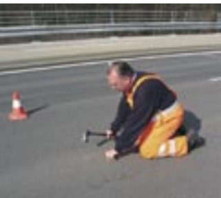
Debonding of asphalt.
