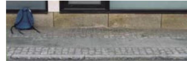
Spalling of granite surface due to rust formation.
