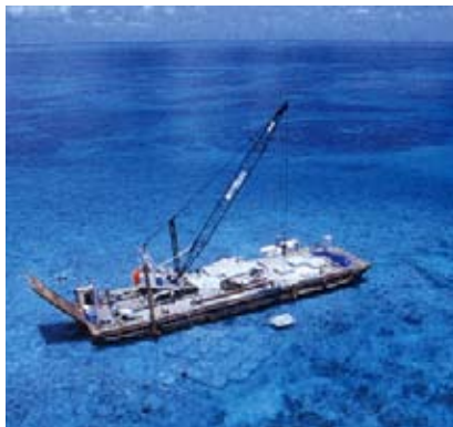
Installation of pre-cast concrete panels for the repair of damaged coral reef
